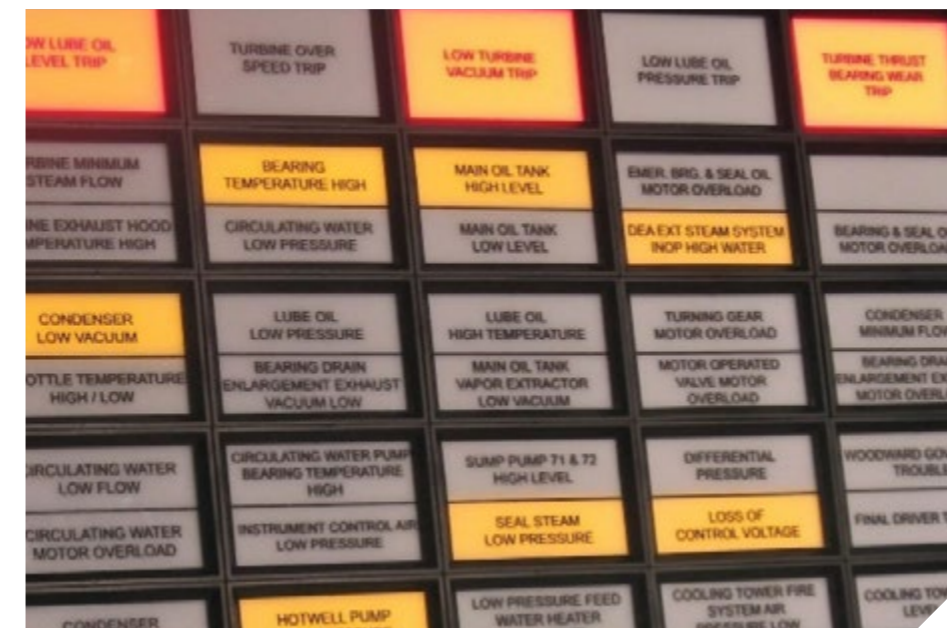
A typical annunciator panel found in machinery control panels and in plant control rooms. At one time, interfacing to such panels was done primarily by means of relay contacts. Today, it is more common for digital protocols to be used for sending status and values to the control room, whether directly to DCS screens or to an annunciator panel.
